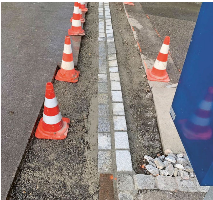
Randstein Reperatur Wingerstrasse, Salez
